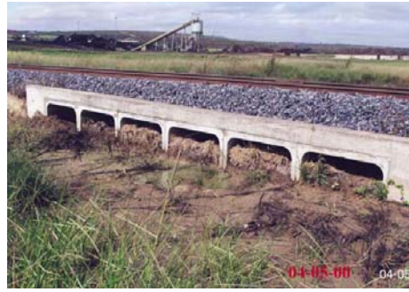
eroded sediments chocking culverts
