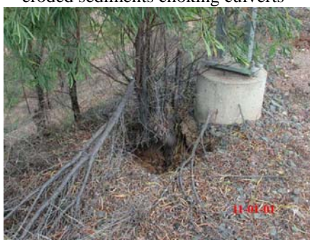
tunnel erosion inlet undermining mast foundation on an embankment
