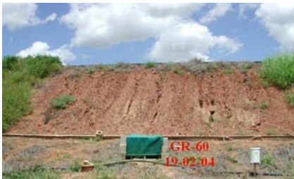
control plot – rill, inter-rill & tunnel erosion occurring
