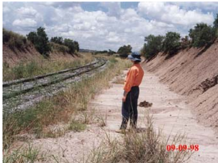
eroded sediments fouling ballast in a cutting
