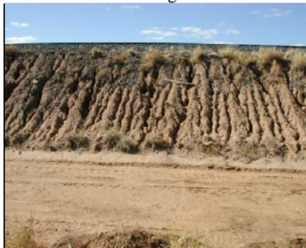
eroded sediments chocking culverts
