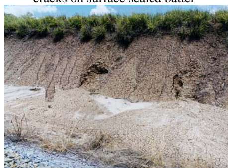
tunnel erosion outlet sediment fans
