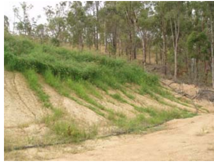
Fig. 14. Holmes cutting – four rows (1 m spacing) of drip lines were laid at the top section only.
